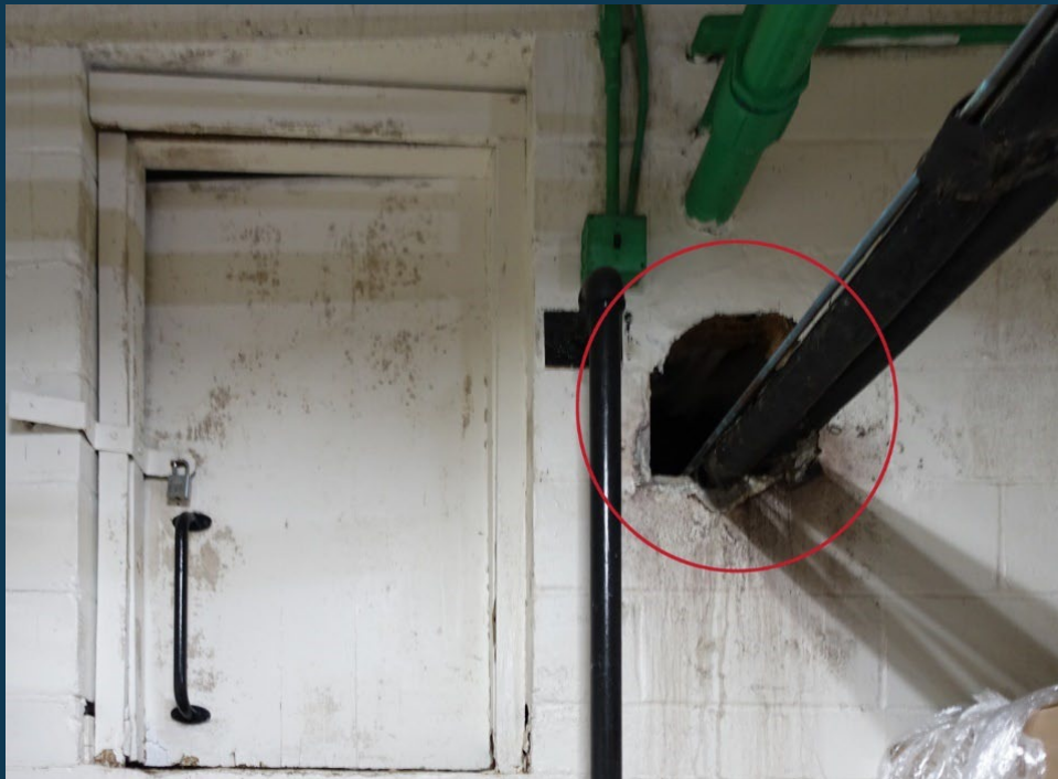
A large open hole in a wall surrounding a pipe's entrance into the food storage warehouse could allow for the entry of insects and rodents.
