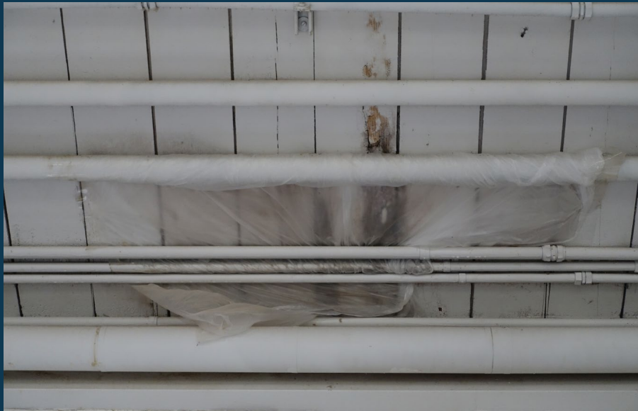
Evidence of Water Intrusion from the Roof, with Plastic Covering a Single-Level Housing Unit Ceiling
