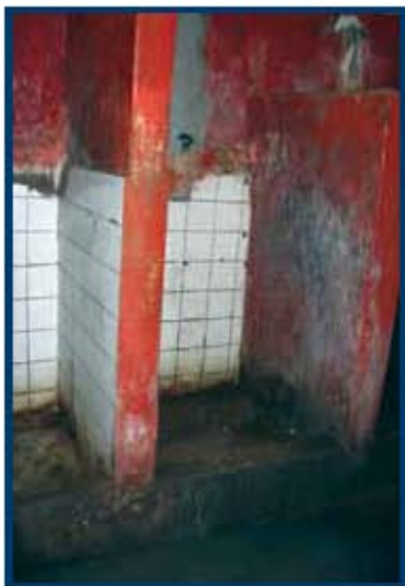
Unsanitary cell block toilets (West Africa) - 2007
