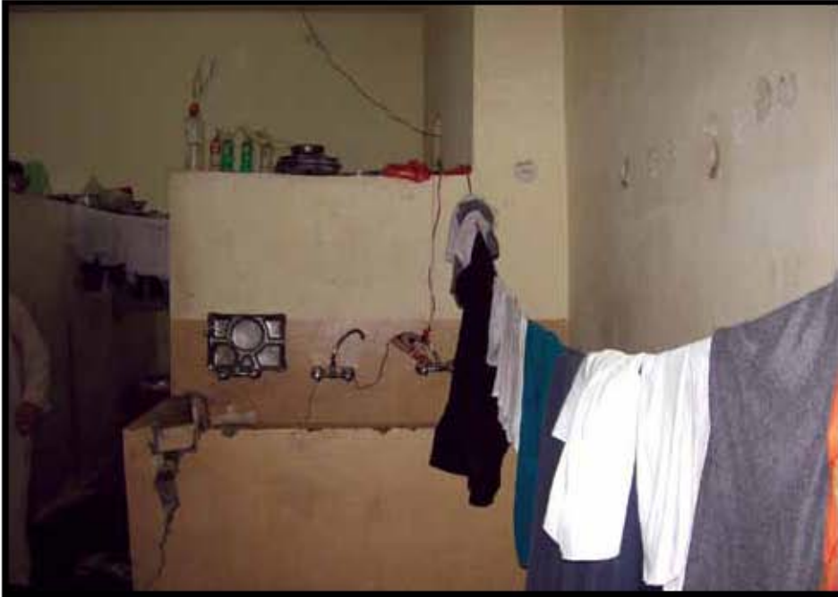
Dilapidated Cell Block Sink (Middle East) - 2005
